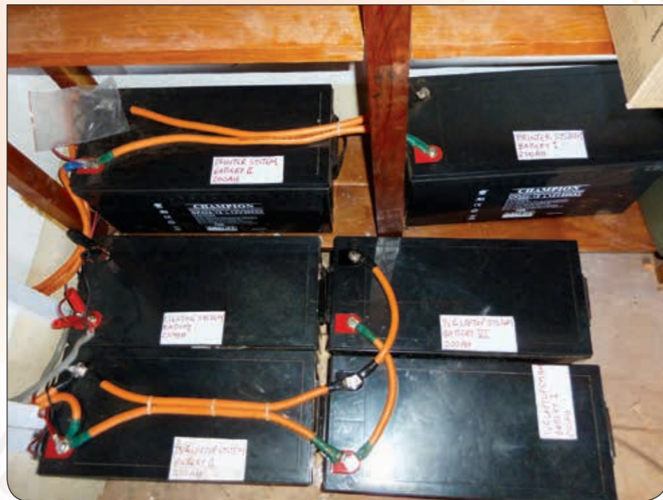
The batteries for the TV, IT and lighting systems at the Energy Centre
